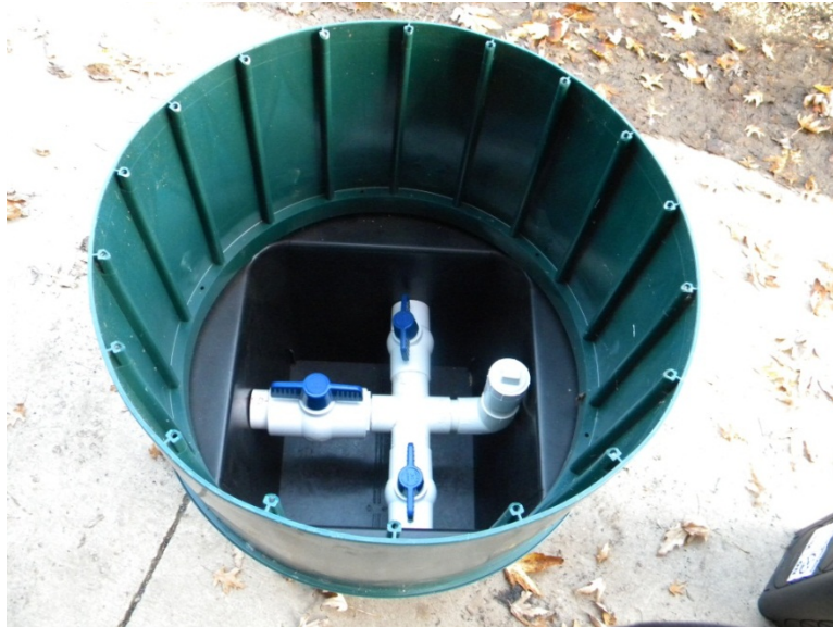
Figure 7. Service box within the manifold line
