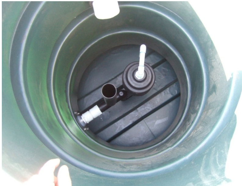
Figure 6. Dosing siphon - internal view
